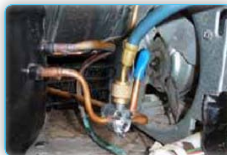
Bullet valve clamped on pipe
