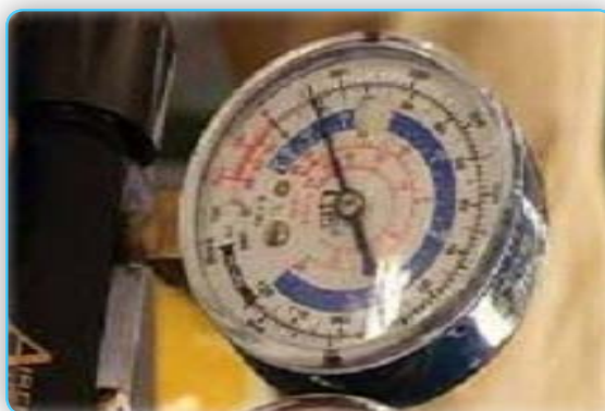
Refrigerant pressure displayed on the recovery gauge
