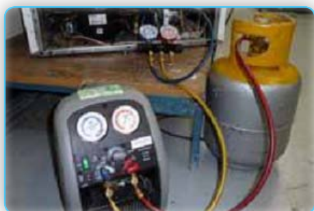
Refrigerant recovery unit and service hose setup
