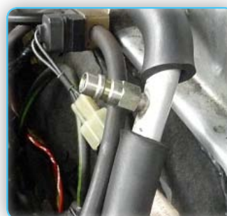
R134a access point
